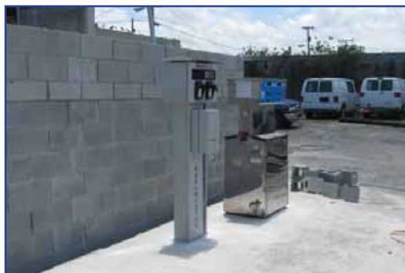
First Compressed Natural Gas (CNG) Station in Florida.
